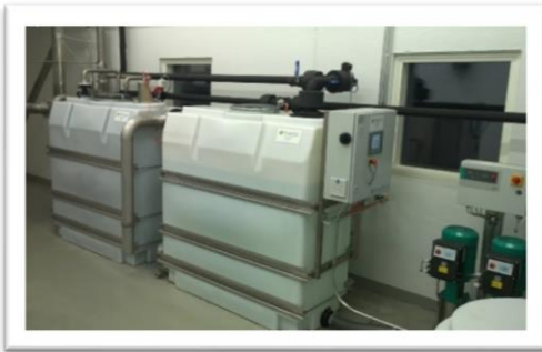
Waste water heat recovery system
